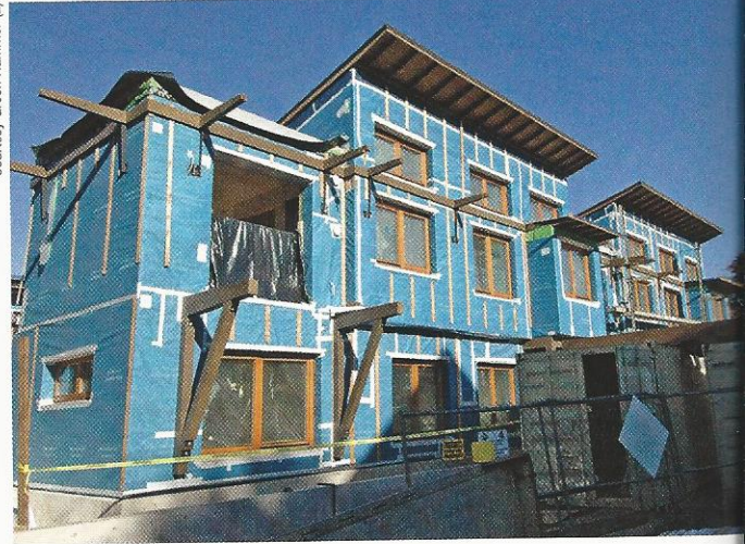
The moisture and air barrier is SIGA Majvest woven polyolefin, which helps keep air leakage under 1.00 ACH 50.
